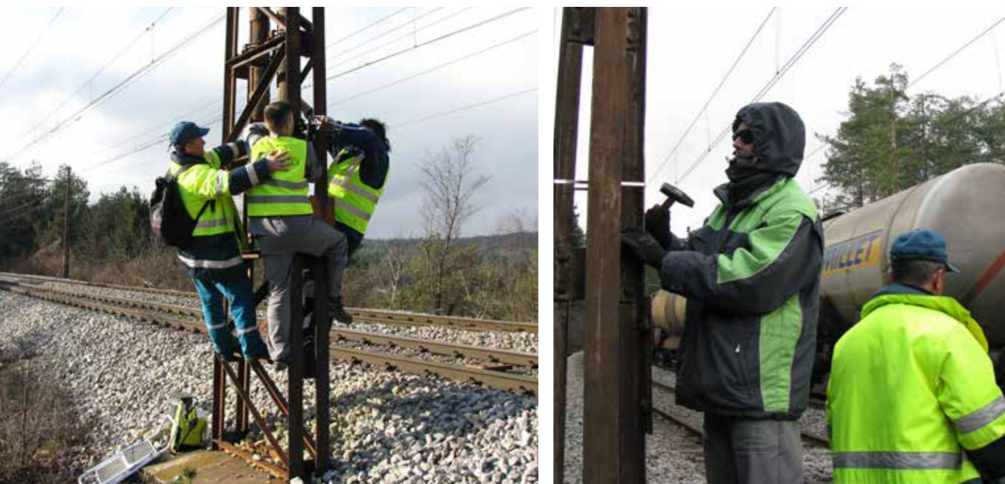
Positioning sound deterrents at critical sections of railway line Rakek – Postojna and Postojna – Prestranek. (Zaluberšek M.)
