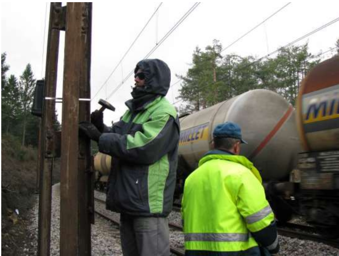
Figure 8: Installation of acoustic deterrents on electric poles along railway sections (photo: M. Zaluberšek, 2015).
