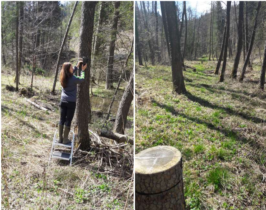
Figure 35: Installation of IR cameras at Ortnek and sensors in wooden stumps capable to detect large animals approaching the roadway (photo: Z. Pavšek, 2017).
