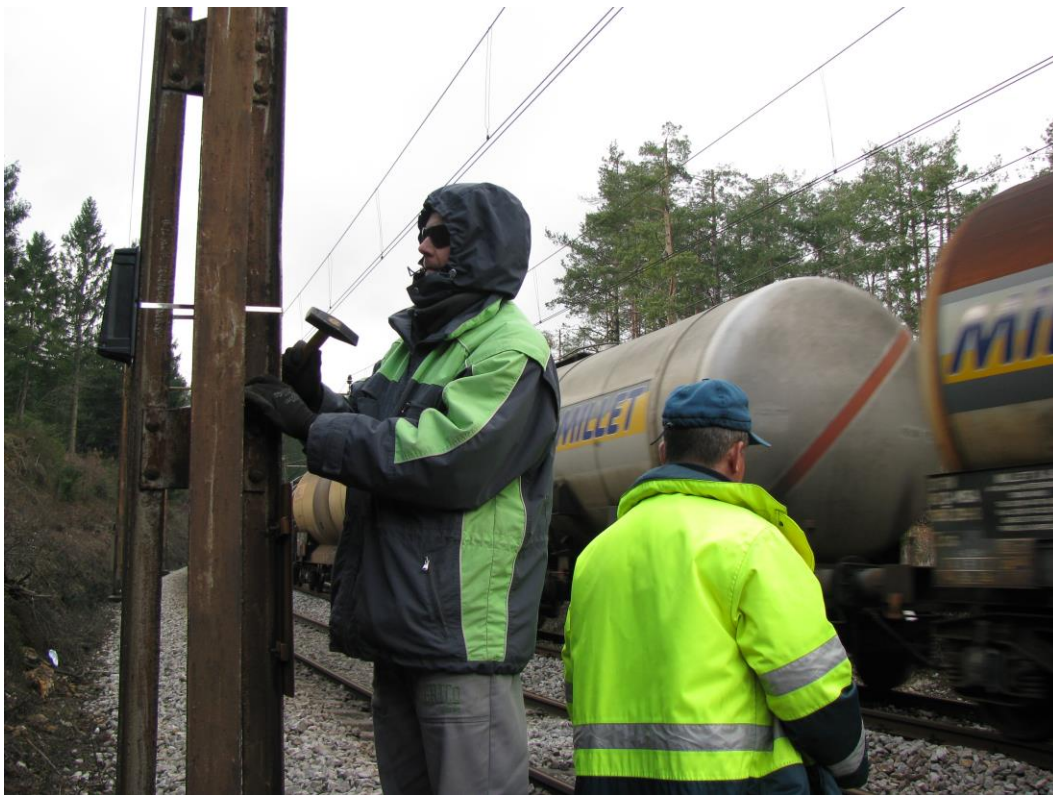
Figure 5: Installation of acoustic deterrents on electric poles along railway sections (photo: M. Zaluberšek, 2015).
