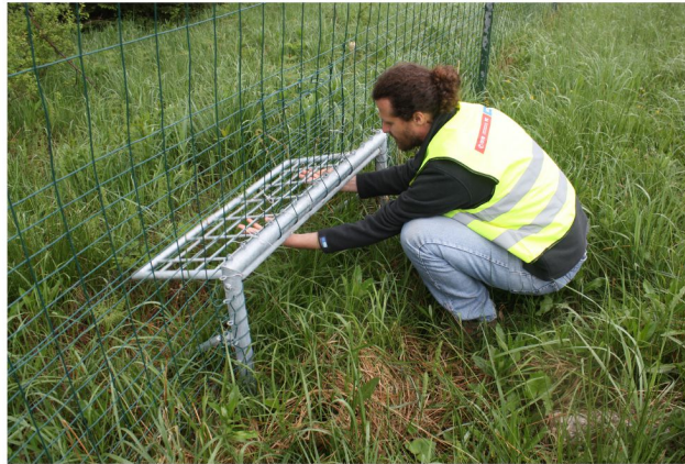
One-way door for animals to exit the highway corridor. Small door.
